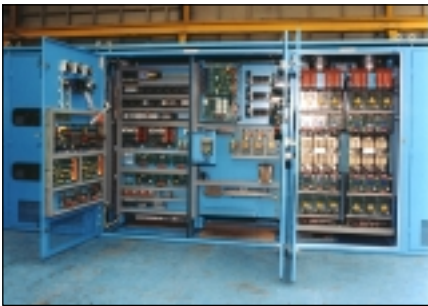
One of the three "Synchrosil" air-cooled variable-frequency drives for each vessel.
