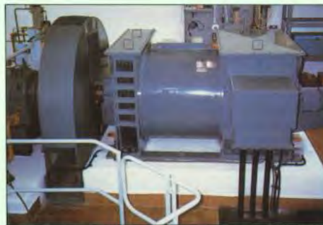
Fig. 12 One of the two Brush 600 kW, 750 rev/min (overspeed 1350 rev/min), 415 V, 3 ph, 50 Hz, generators installed in the Sulby Power Station, Isle of Man, U.K.
