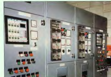
Fig. 28. Combined L.V. switchgear, control gear, and protective relay panel for two induction generators rated at 696 kW and 318 kW supplied through Gilbert, Gilkes and Gordon for installation at Littlewood River, Idaho, U.S.A.
