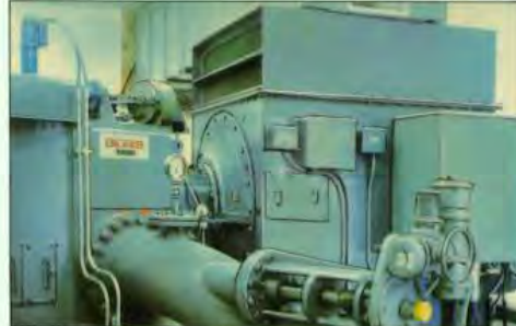
Fig. 9. Brush 1.976 MW, 514 rev/min (overspeed 1000 rev/min), 4160 V, 3 ph, 60 Hz, generator installed at the Dillon Dam Hydro Site, Denver, Colorado, U.S.A. Machine supplied through Gilbert, Gilkes and Gordon, and Hawker Siddeley Power Engineering Inc.
