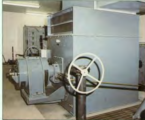
Fig. 8. Brush 1.9 MW, 720 rev/min (overspeed 1225 rev/min), 4160 V, 3 ph, 60 Hz, generator installed at the Bidwell Ditch Hydro Scheme, Redding, California, U.S.A. Machine supplied through Gilbert, Gilkes and Gordon and Mega Renewables.
